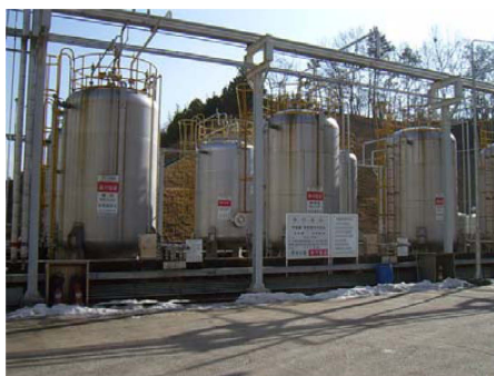
Storage tank of solvents
