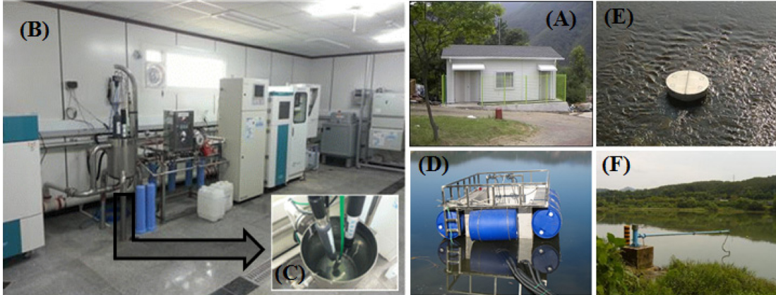
Fig. 2. Monitoring system and sampling facilities (A: the monitoring station, B: inside the monitoring station, C: measurement system by using YSI 6600 in storage tank, D-F: barges, manhole, and bridge piers types sampling system).
