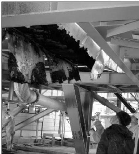
Fig. 1. A part of seriously corroded desulphurization system in Yeosu power plant.
